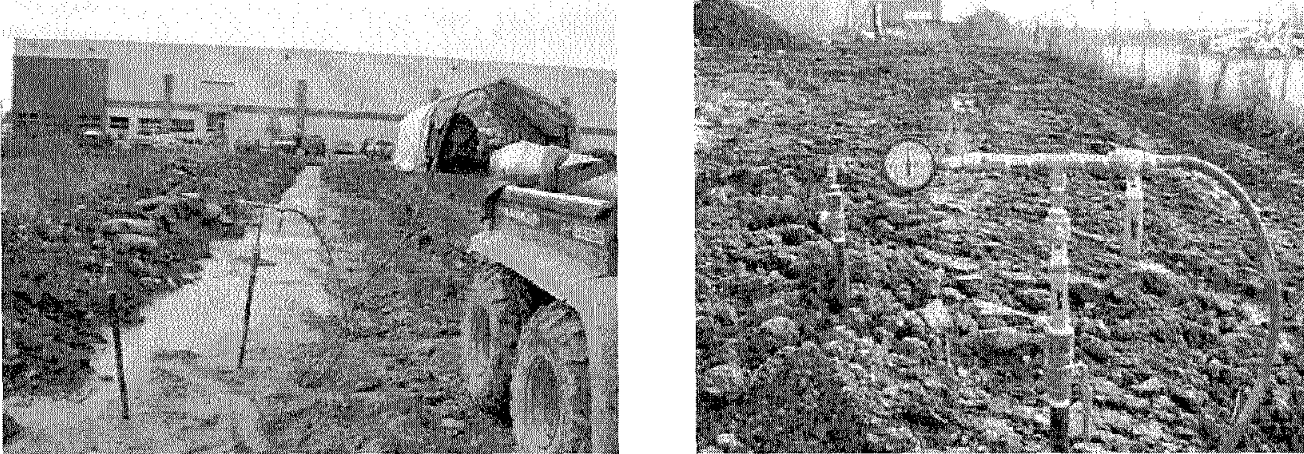
Figure 3: Representative illustrations of installed PA12 pipe segments using both (a)flowable fill and (b)rock soil mixture
