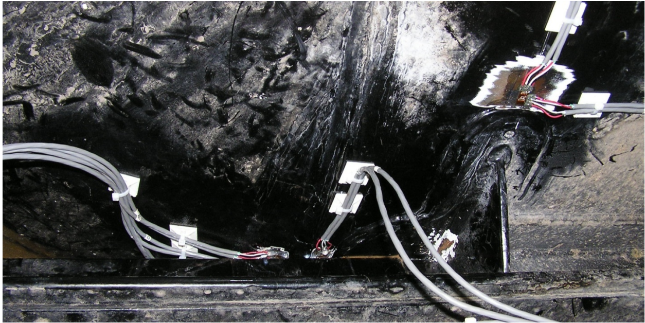
Figure 7. Underside of tank showing the weld pad and one of the six pad-to-tank rail gusset.
