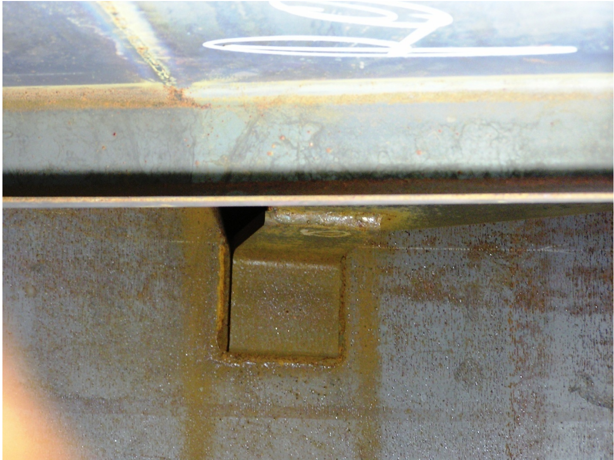
Figure 5. Tank internal baffle and baffle attachment to tank wall.
