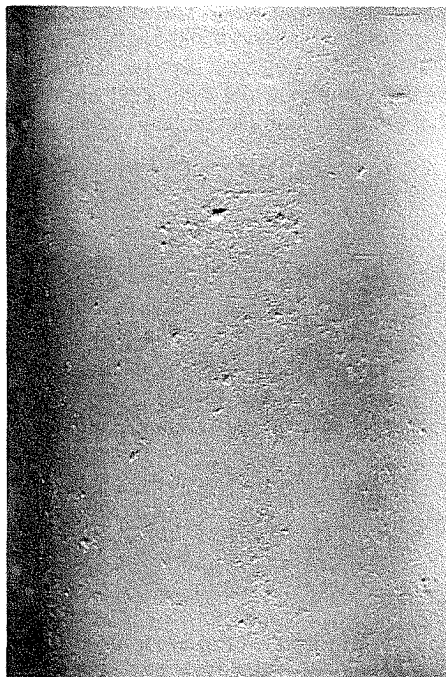
Figure 5—General corrosion with isolated pitting on cylinder sidewall
