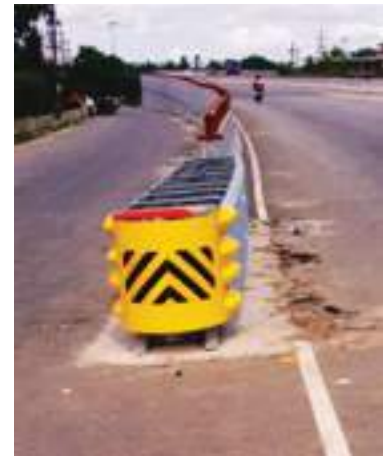
Impact Attenuators at gore areas having high speed traffic bifurcation
