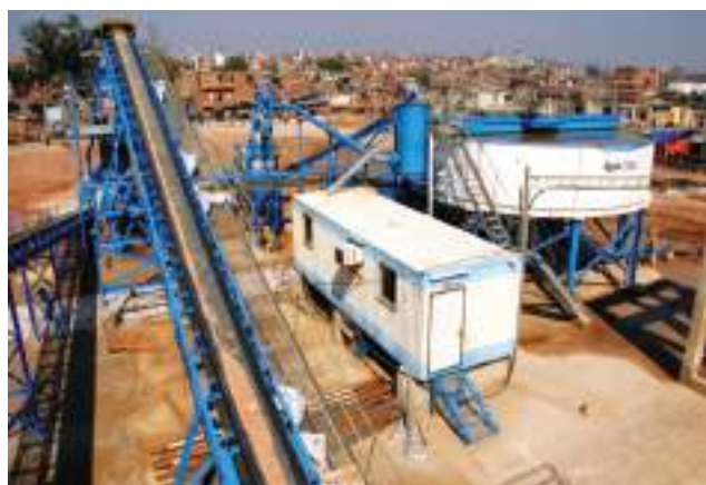
Photo 4 C&D Wet Processing Plant
