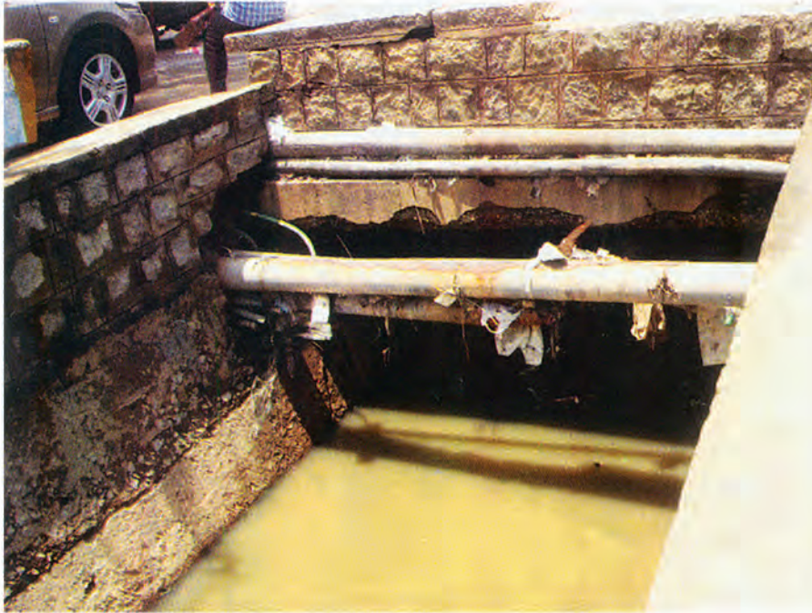
Photo-10 A Sample of Debris Clogged Due to Passing of Utility Lines in
