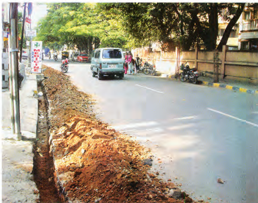
Photo-11 A Sample Photo of Recently Laid Surface Opened Due to Lack of Coordination
