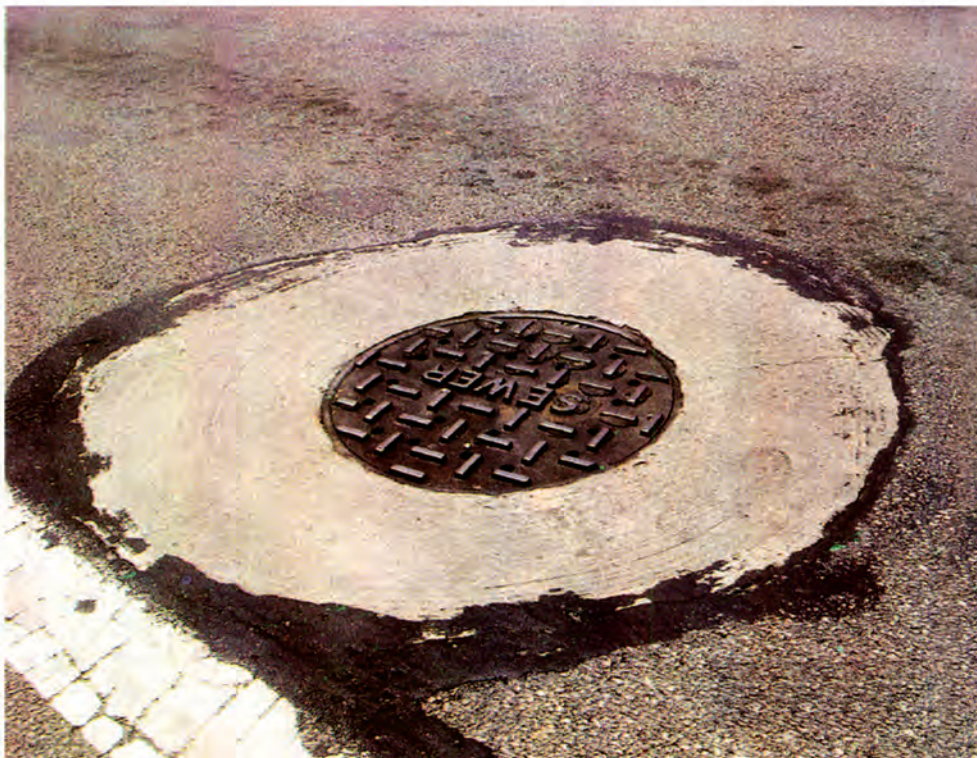
Photo-3 A Sample Photo of Damaged Manhole Cover
