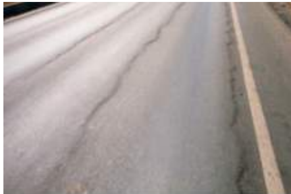
Photo 7.4.4 Shoving of Bituminous Surface
