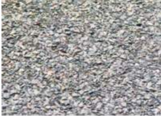
Photo 7.5.1 Stripping of Bituminous Surface
