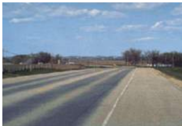
Photo 7.4.7 Upheaval in Bituminous Surfacing
