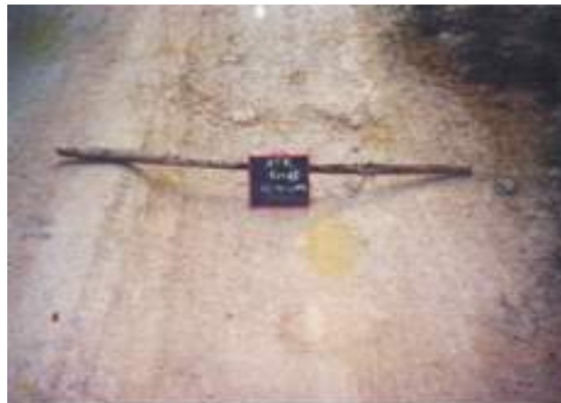
Photo 7.4.6 Settlement in Bituminous Surfacing
