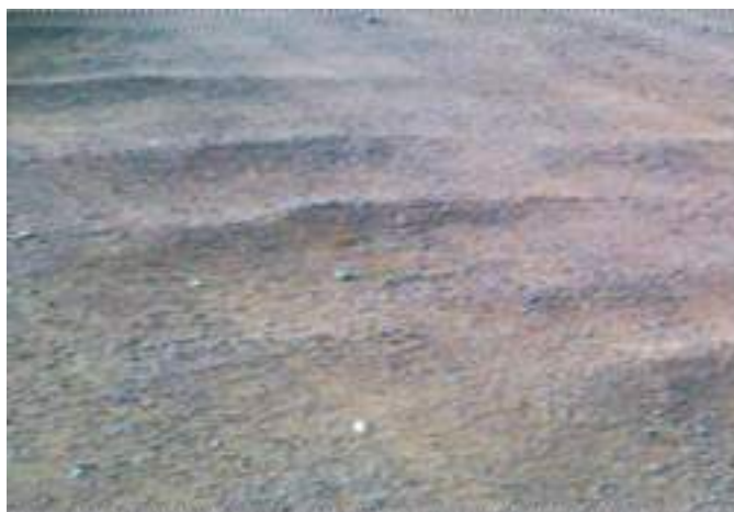
Photo 7.4.3 Corrugation of Bituminous Surface
